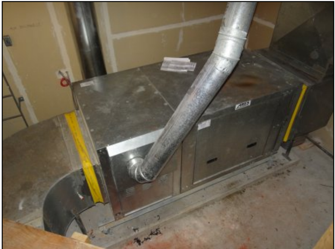
Natural gas-fired make-up air unit observed in the attic of each building.
