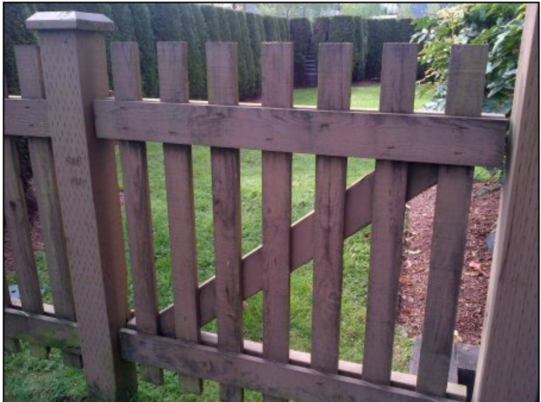
Some deterioration of paint coating observed on wood fencing.
