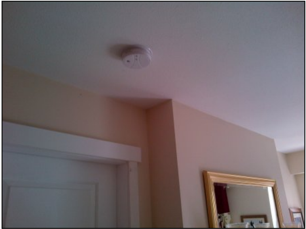
Smoke detectors observed in suites.
