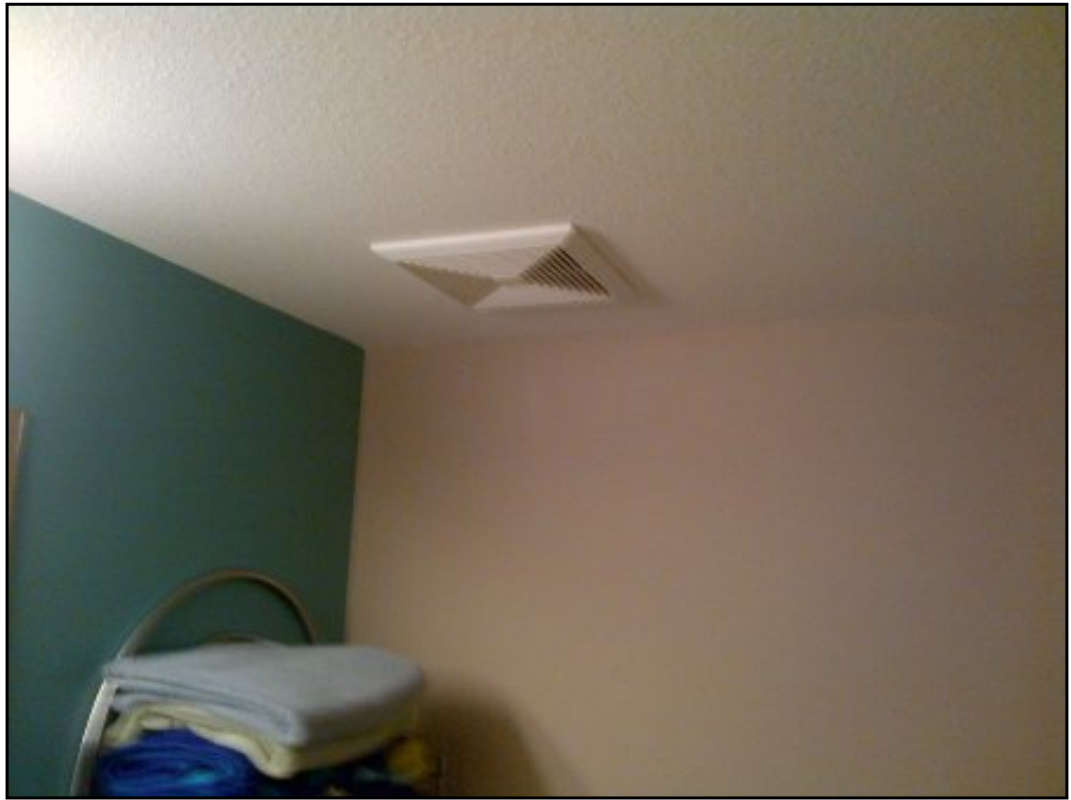
Exhaust fan observed in washrooms.
