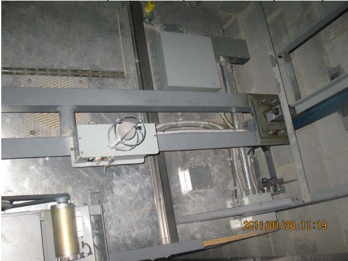
Photo 9 – Elevator 2 Car Top at 400 Klahanie (300 & 500 same except no car top railing)
