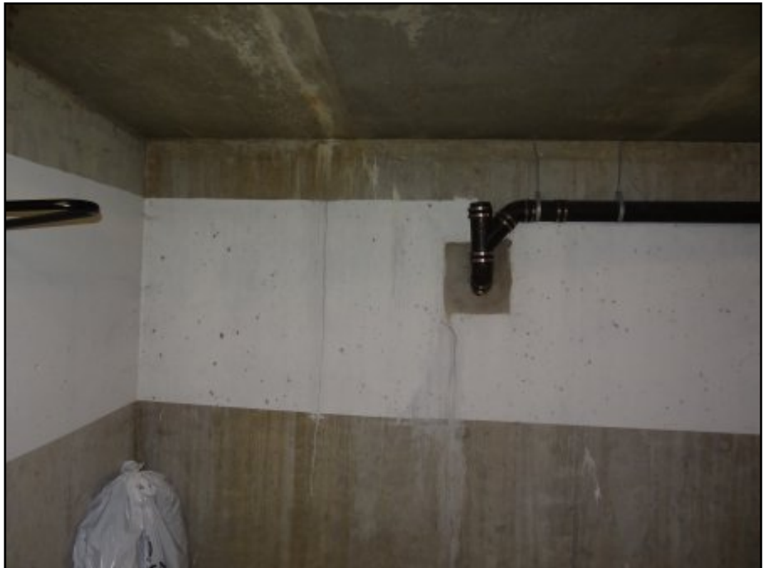
Cracks observed on foundation walls in parkade.
