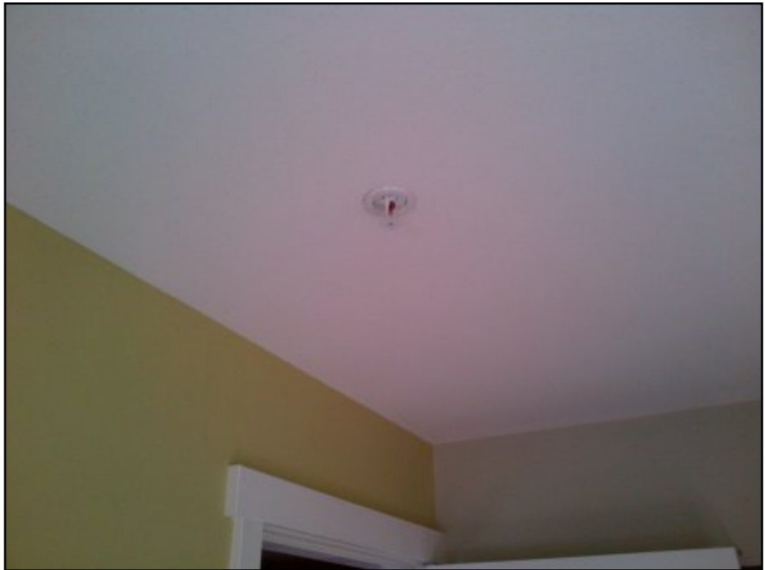
Sprinkler heads observed in suites.
