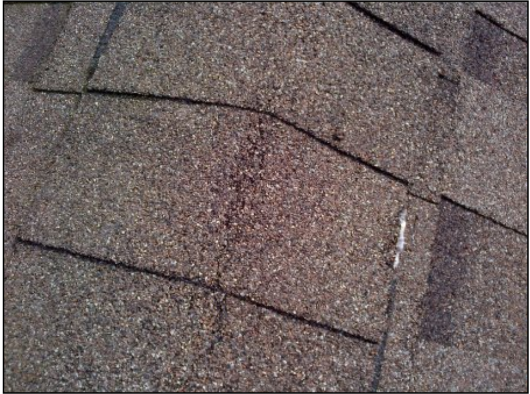
Cracked shingles observed at roof peaks.
