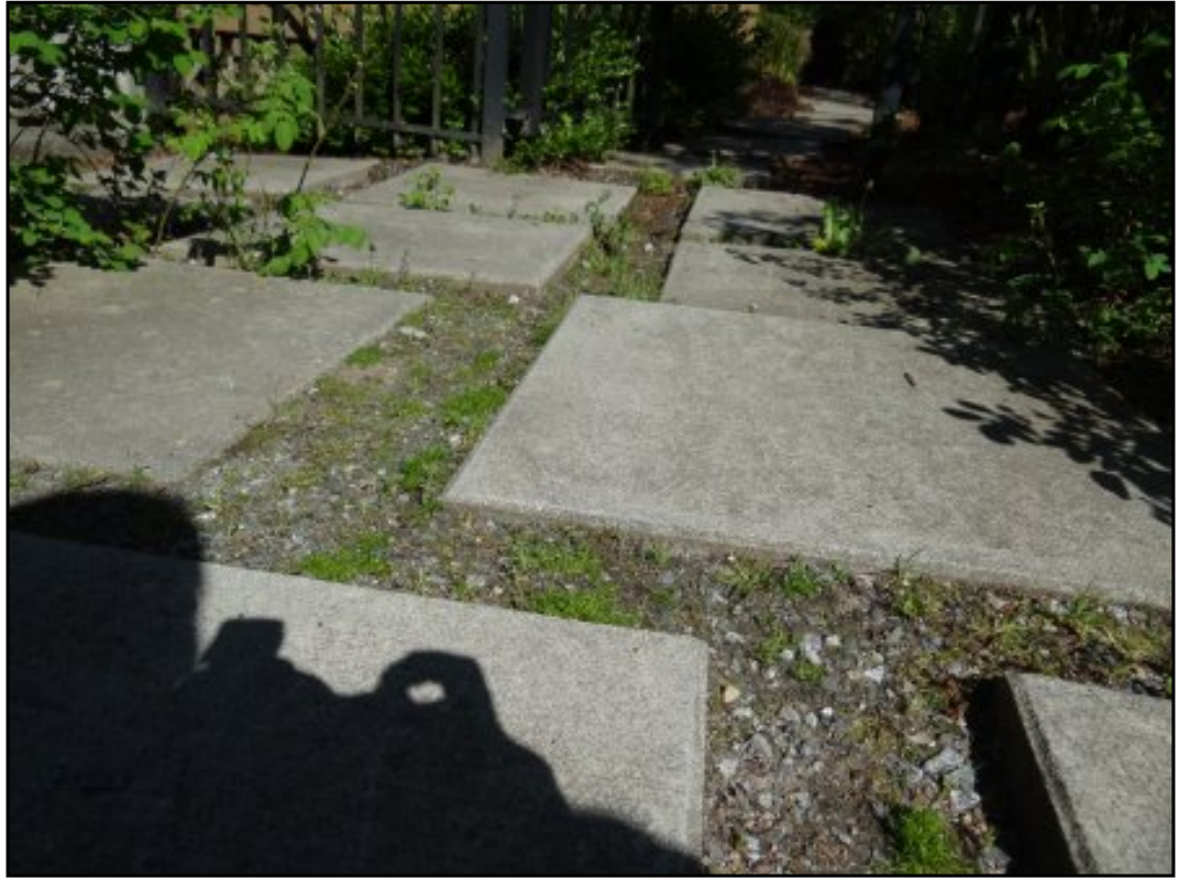
Eroded soil around paving stones between Buildings 300 and 400.
