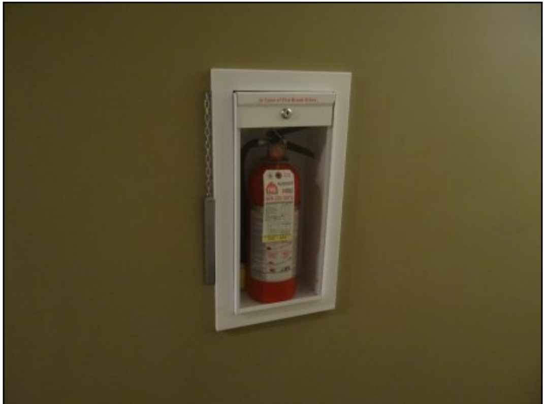
Fire extinguishers observed in hallways.
